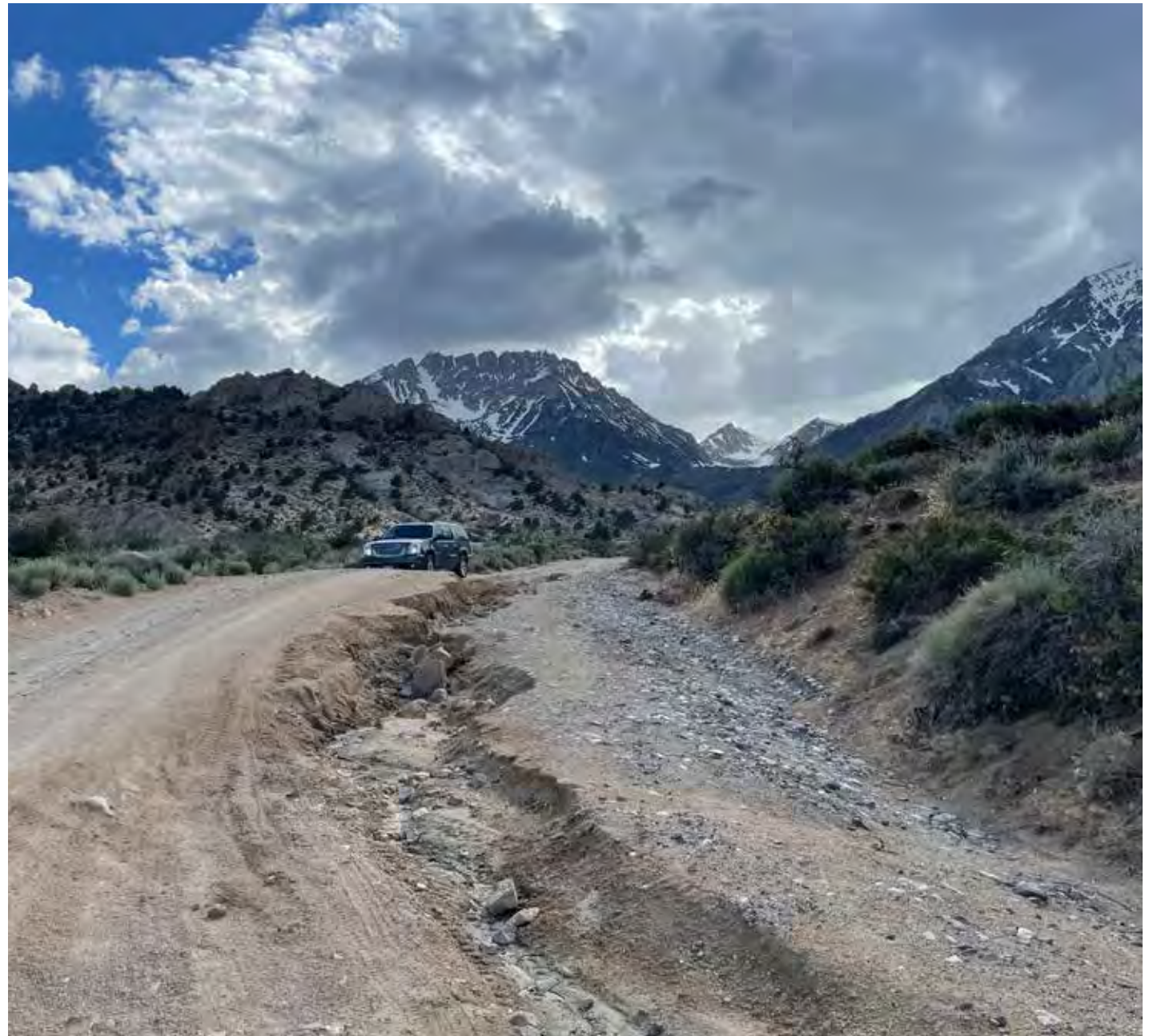
Because Buttermilk Road has not been regraded, the existing drainage systems have been made ineffective.
