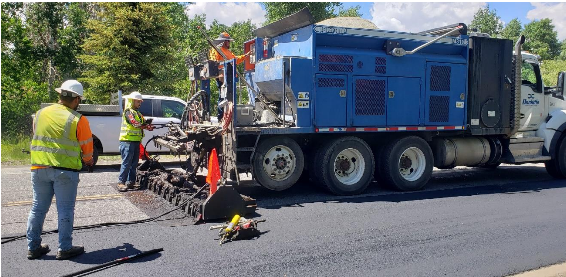
The specialized box truck required for a slurry seal. The machine mixes sand, aggregate and oil before laying material at a precisely measured thickness
