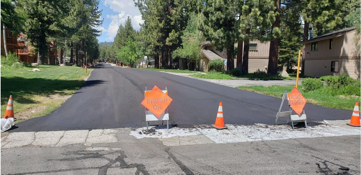
A fresh seal along Azimuth Drive. The surface could typically be driven over within 10-15 minutes
