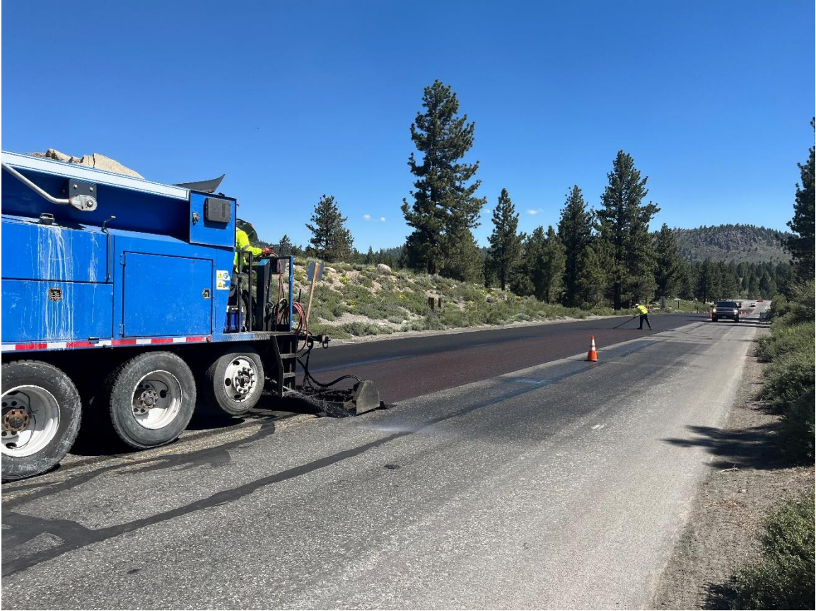
Traffic continuing to pass along Meridian Boulevard while another coat is layed in the middle lane
