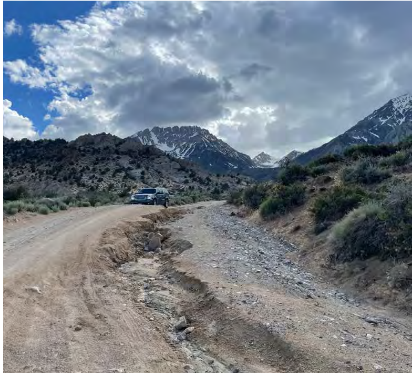
Because Buttermilk Road has not been regraded, the existing drainage systems have been made ineffective.
