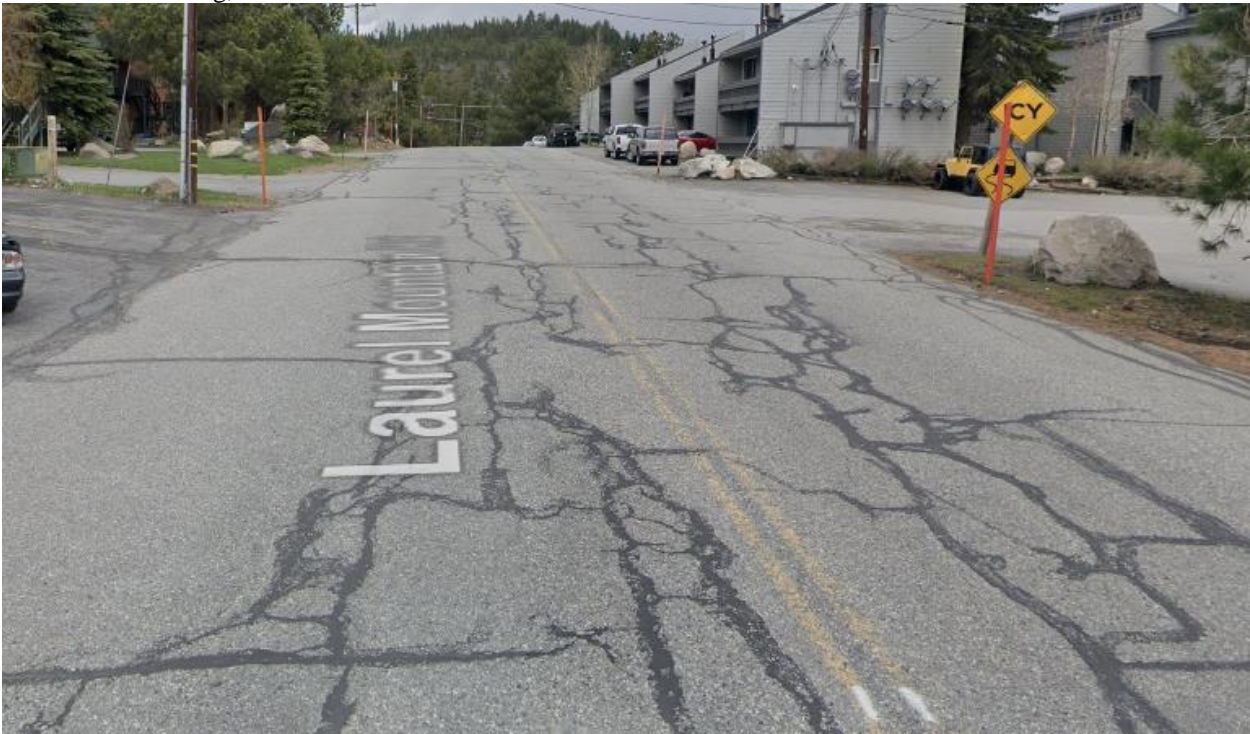
Severe road cracking, no sidewalk
