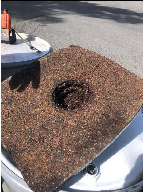
Internal corrosion buildup
