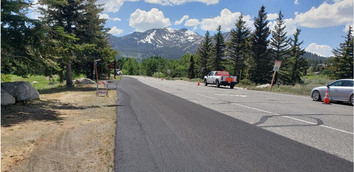
Old Mammoth Road with a fresh coating (left) vs the existing asphalt condition (right)
