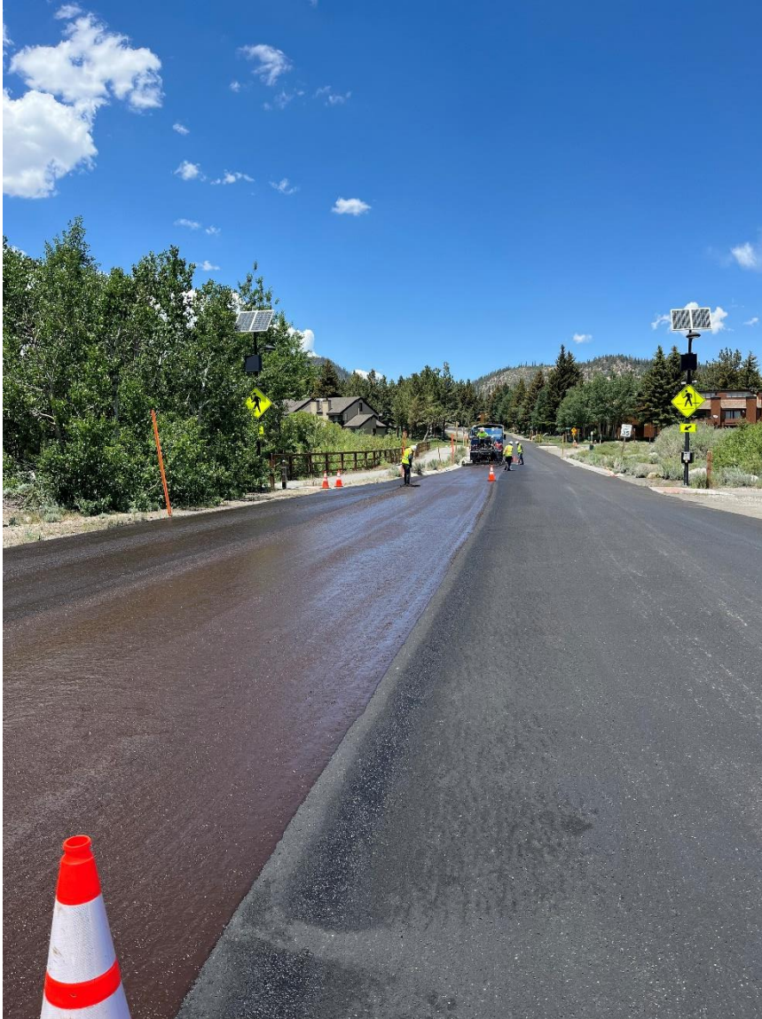
A wet slurry (left) adjacent to a cured slurry (right). These two coats were likely laid within 1 hour of each other
